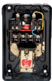
Interior View of MK1 DOL
