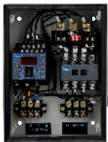
Interior View of MD Starter+ DOL Starter
