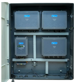
Interior View of xMasm10 - Wired Solution
