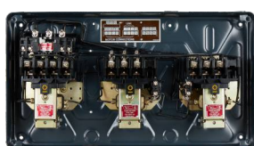
Interior View of MK1 SASD
