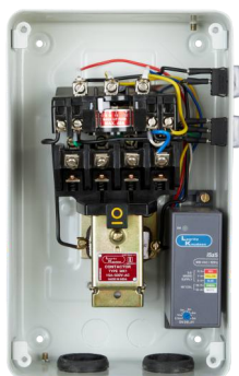
Interior View of MK1.i
