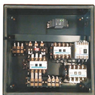
Interior View of MU-G20W FASD
