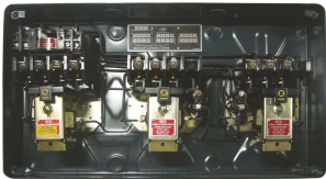
Interior View of MK1 SASD
