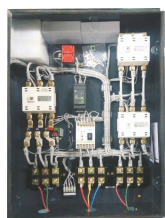
Interior View of MU-G30W FASD
