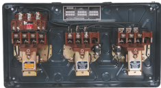
Interior View of MK2 SASD
